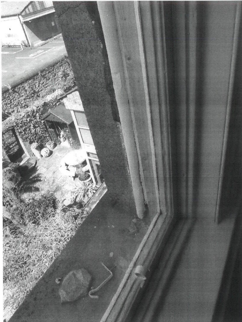
Photo 5 – Window to rear, note failing external reveal with debris on sill, and prop to upper sash (broken cords)
